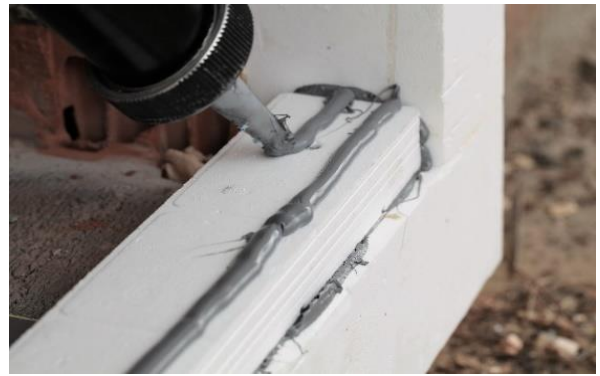
Photo 20 – Application of a hybrid to the BP beam; arrangements for joining the BP beam and the frame
