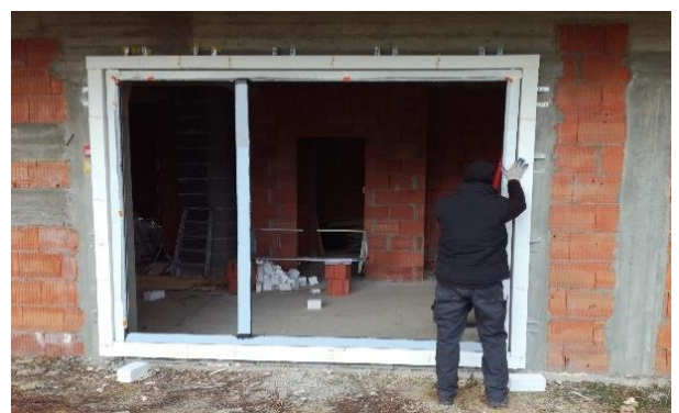
Photo 22 – Stabilisation of the frame with wedges prior to drilling holes and screwing the head in
