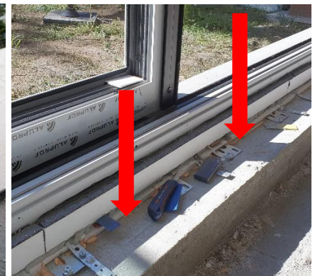
Photo 20 – Non-recommended application of plastic washers
