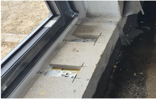
Photo 5 – Cutting and chamfering of ferroconcrete sill. Embedding of CBM bracket sheet plate at a required level
