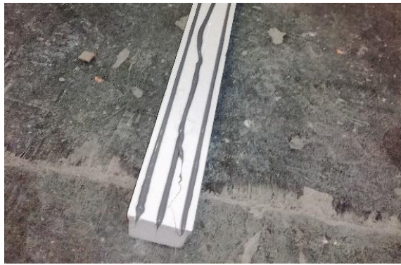
Photo19 – Three doses of a hybrid on the BP beam; joining the BP beam and CBM beams within the under-window zone
